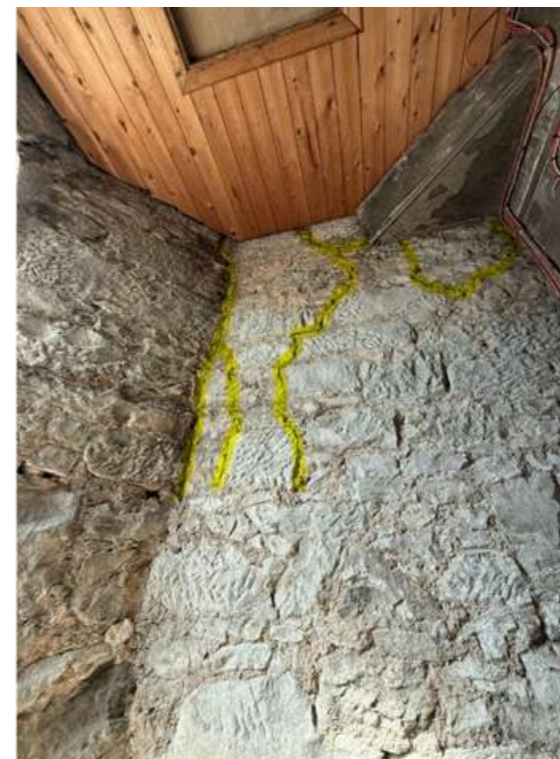
Figure 3 – Crack formations on the western facet (highlighted in yellow)
