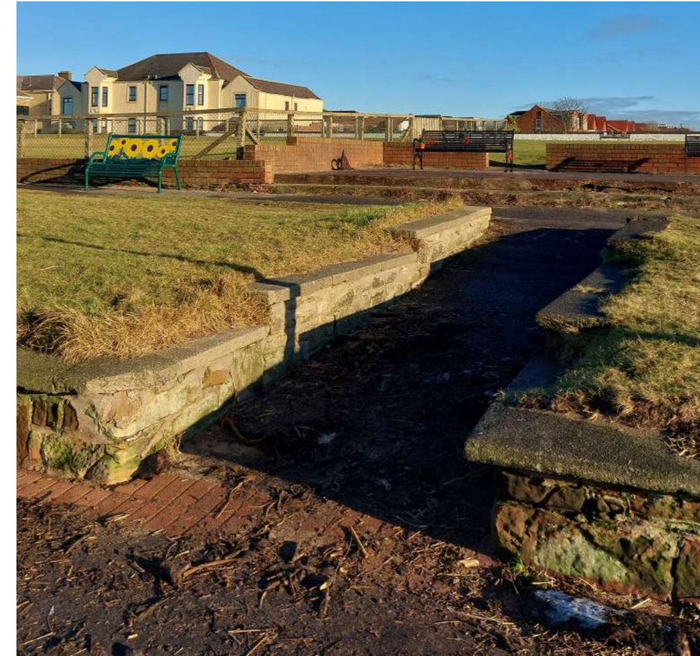
Difficult to maintain materials and details
