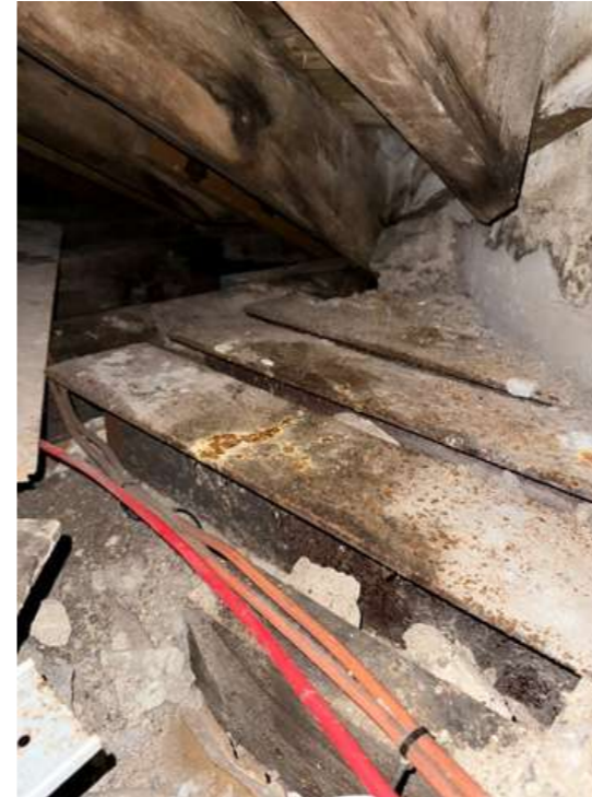
Figure 2 – Corroded Steel Beams supporting the tower
