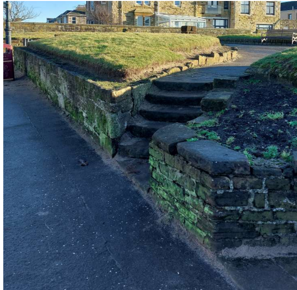
Poor quality accessibility
