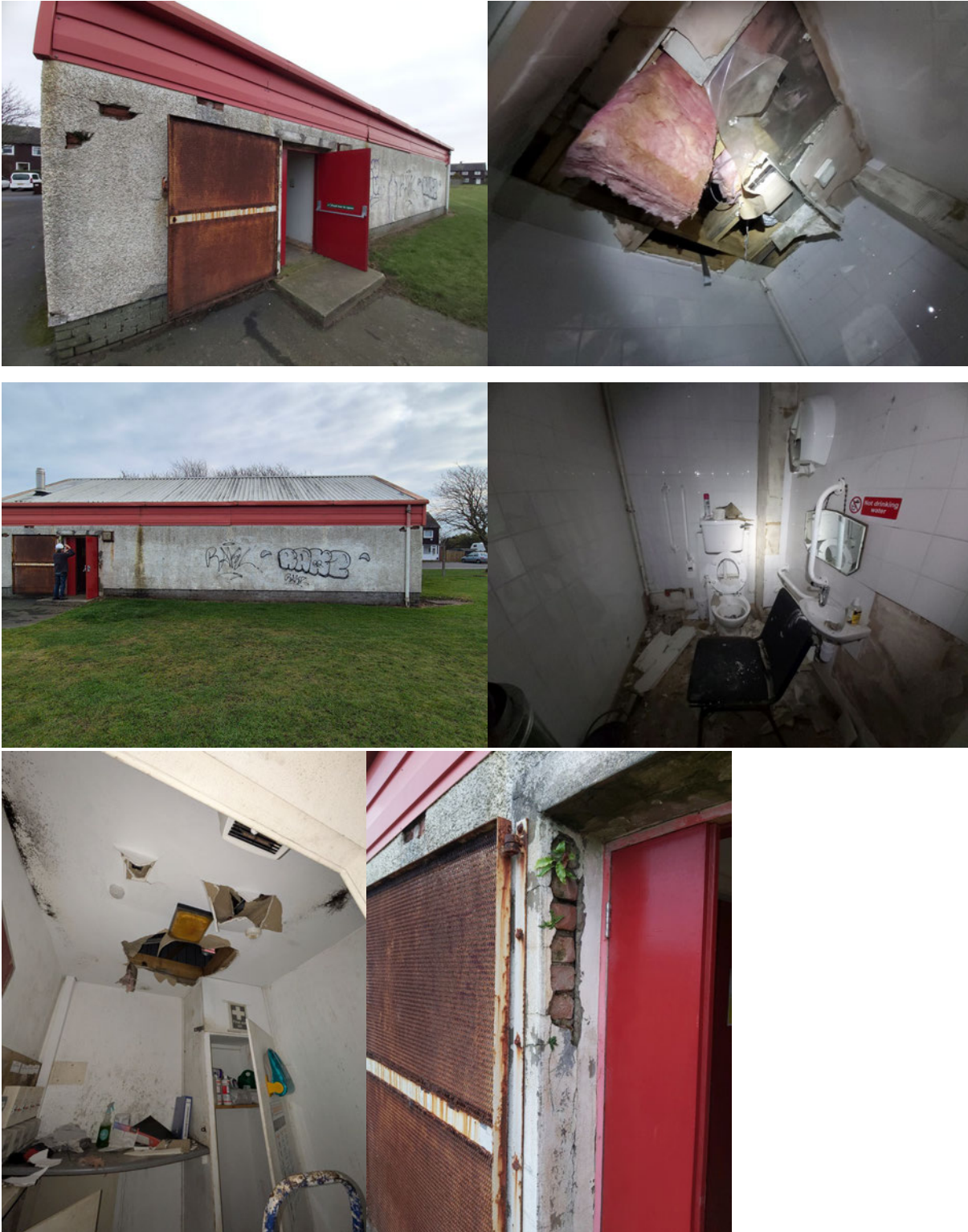
Figure 8: Current condition of Hosiery Park Pavilion
