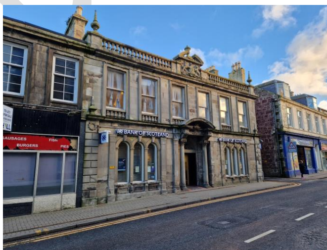
Stonework Erosion, 17 Dalrymple Street
